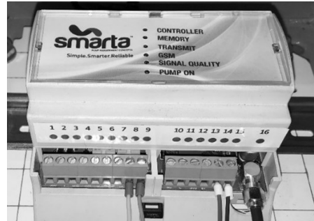
Figure 6 SMARTA Logger terminals
