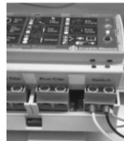
Figure 8 Pump control box/panel switch input
